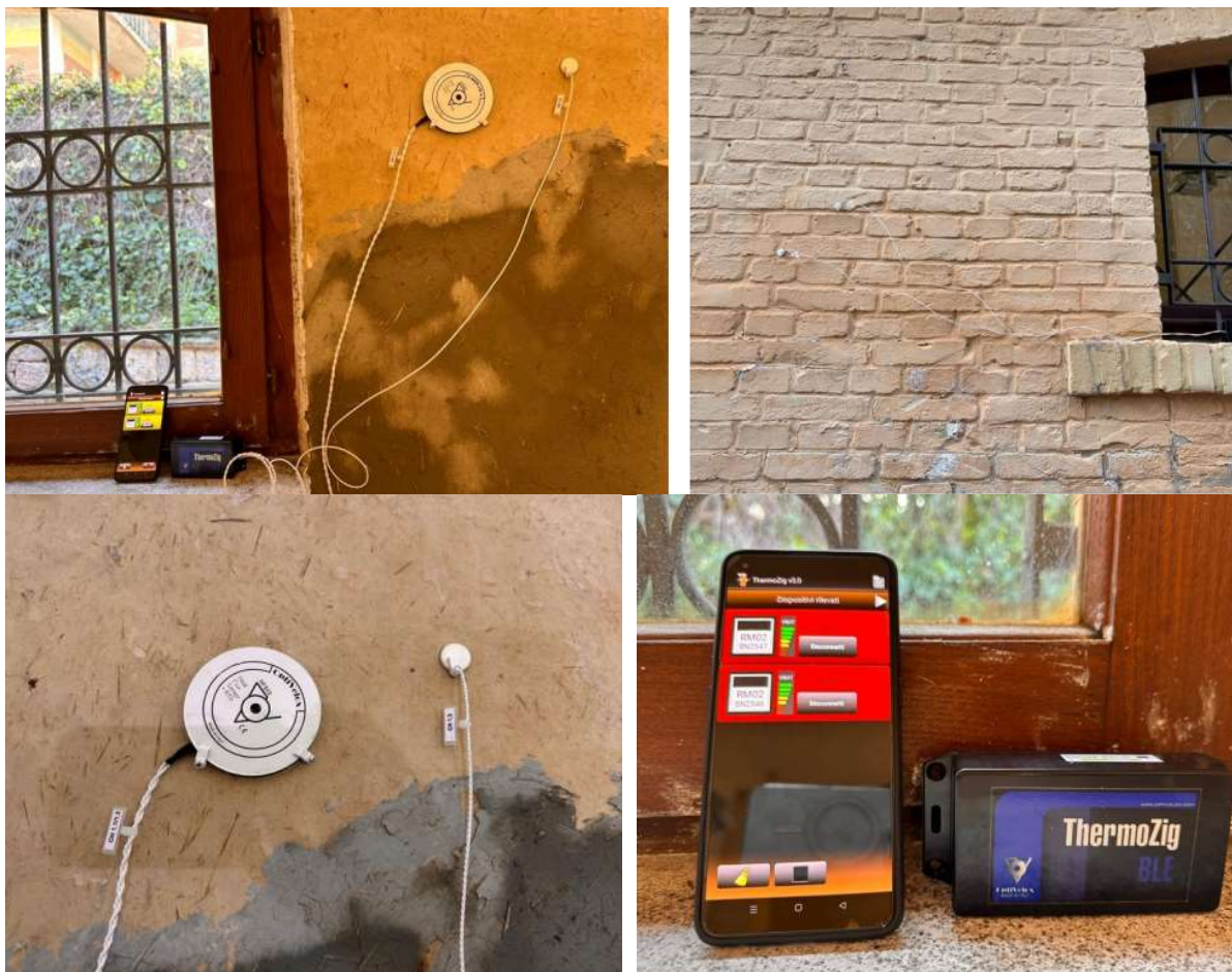
Fig. 14 Thermal flux meter for thermal transmittance evaluation.
